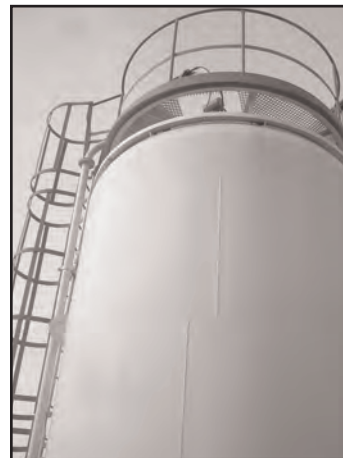
Flexar™ technology on lime silo
