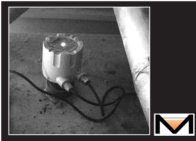
This Model MK-2e is monitoring the level of latex paint.
